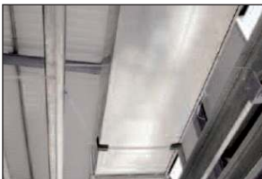
Square Air Ducts
