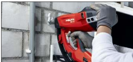
Conduits and light-duty pipes
